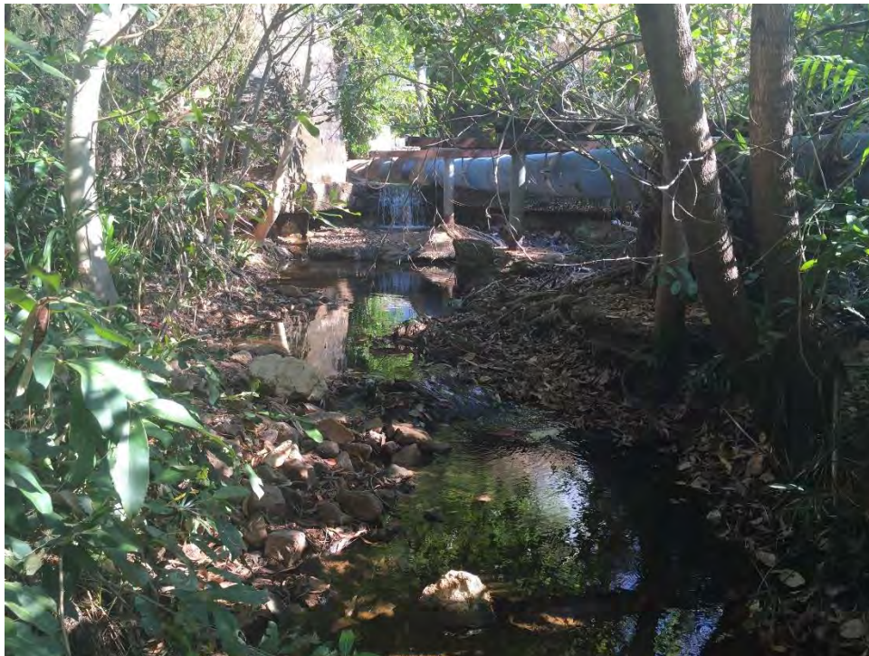
Figure 4-8: Discharge from stormwater pipe to creek from car park to south of site.
