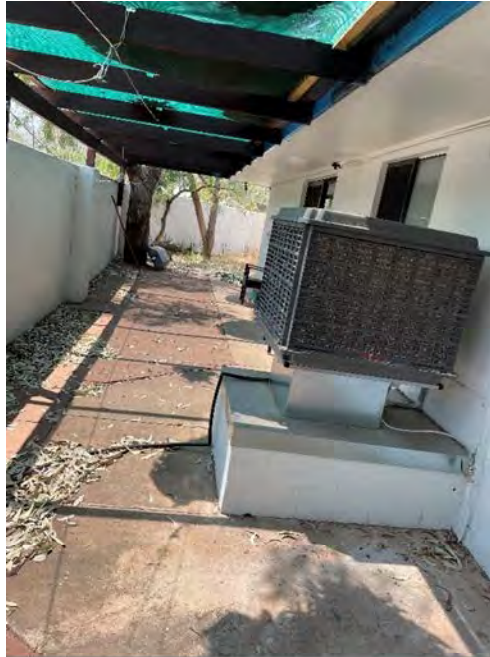
Figure 10 - Managers Accommodation Evaporative Unit
