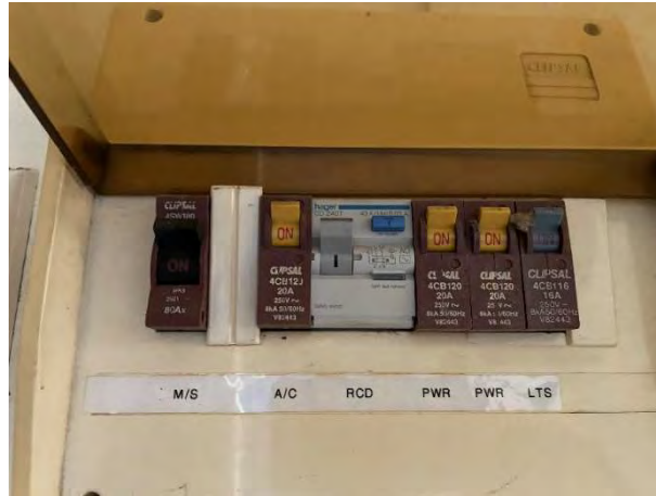
Figure 13 - Switchboard in Single Room / Studio Apartment
