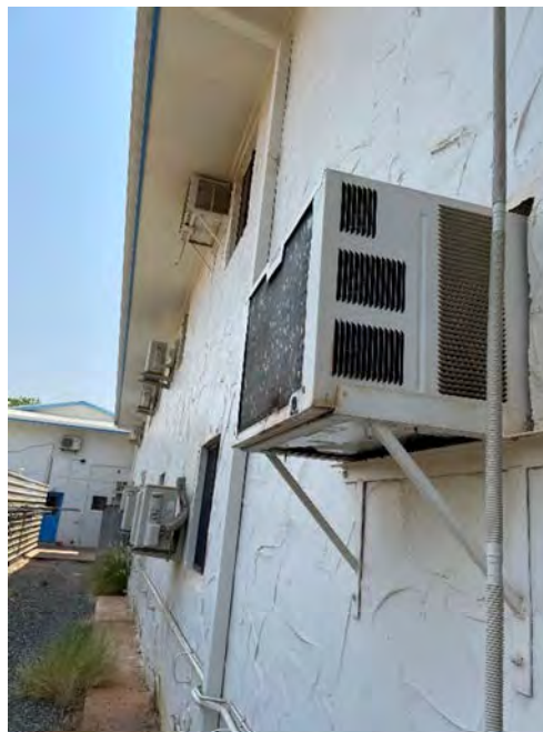
Figure 9 - Outdated and redundant Box type unit
