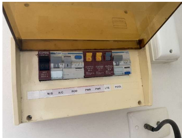
Figure 14 - Switchboard in Single Room No. 4
