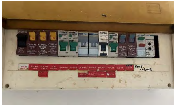
Figure 16 - Switchboard in Reception
