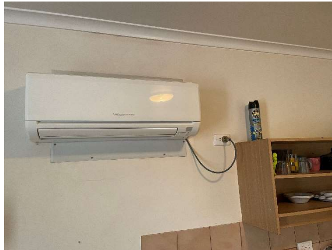
Figure 8 - Incorrect and non-compliant wiring to wall-mount unit
