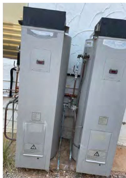
Figure 36 - Existing Hot Water Unit
